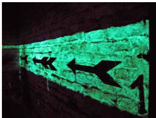
Leuchtfarbe markings directing occupants to the emergency exit. Photo Jonny B Kirchhain
